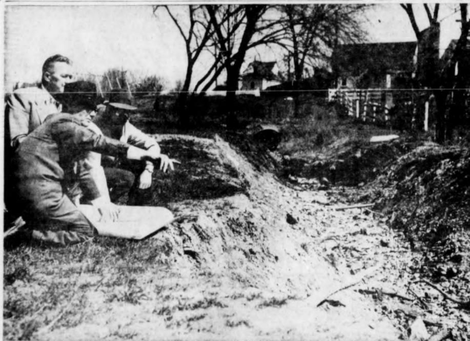
SITE OF DRAINAGE PROBLEM — Soon to be rectified in Leeland Park, Cedar Heights, is pointed out by Oscar Corson, Whitmarsh Township engineer, to John R. Medvetz, 38 Laubert Rd., Andorra Acres, who
