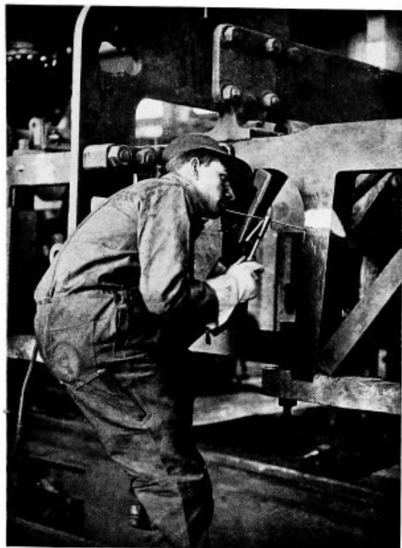
Repairing a broken locomotive frame. The weld, which is shown in white is 3 inches high, 4\frac{1}{2} inches wide, and 4 inches deep. One man finished the entire job in about 5 hours.
