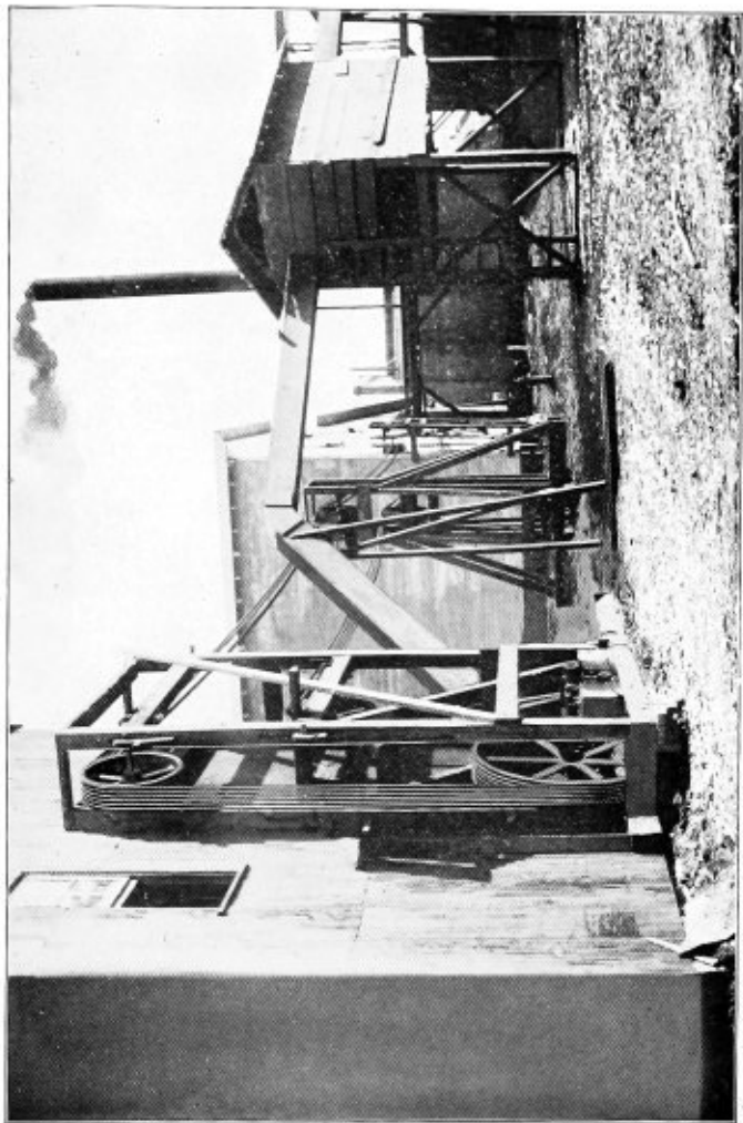
Manila Rope Drive in the plant of the Starkville Cotton Oil Co., Starkville, Miss., transmitting ninety horse power from mill to cotton ginners, a distance of about one hundred and fifty feet. When the power is not required, it is cut off by means of a Weller Standard Friction Clutch.
