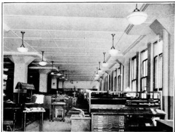
Johns-Manville Acoustical Correction on the ceiling of the Composing Room, New York Tribune. This scientifically designed corrective treatment reduces the annoyance, fatigue and loss of efficiency due to unnecessary sounds, echos, reverberations, etc.
