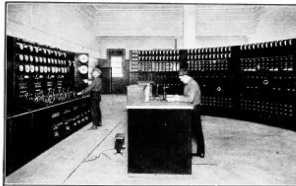
Sections of switchboards at United Electric Light & Power Co., Hell Gate, New York City, one of the most modern power stations in the world. Johns-Manville Ebony Asbestos Wood was chosen for the huge switchboards and many other uses because of its superior dielectric strength, ability to withstand vibration and shock and freedom from metallic veins.
