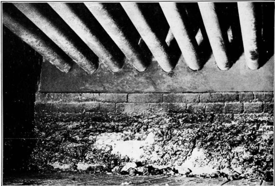
This is an excellent illustration of the Johns-Manville Monolithic Baffle Wall, showing as it does, a solid wall built up around the tubes, with none of the joints and cracks necessarily found in tile baffle walls. It can readily be seen from this picture that leakage of heat-laden gases through such a wall is absolutely impossible, as it is built of a material that will resist and withstand highest temperatures encountered without melting or cracking
