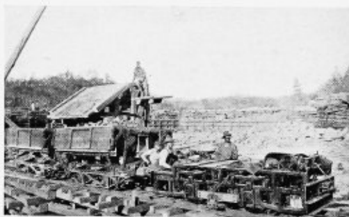
One of six 8-ton locomotives, equipped with motor-driven cable reel, being used in construction work on a dam for a large power project in Alabama. Power is supplied by third rail
